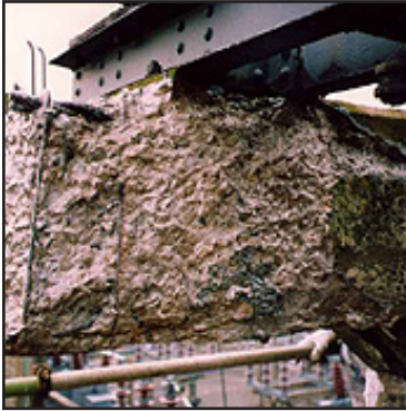
Close up of the badly spalled concrete
