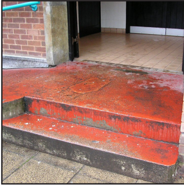
Worn steps were a health and safety hazard
